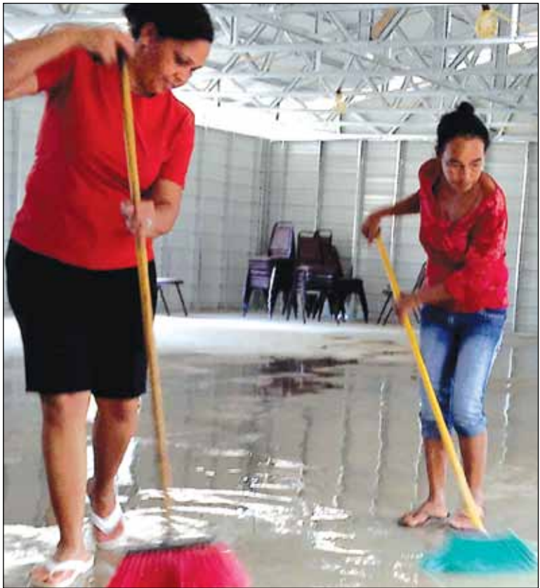
These women spread water over the new floor to keep the dust down.
